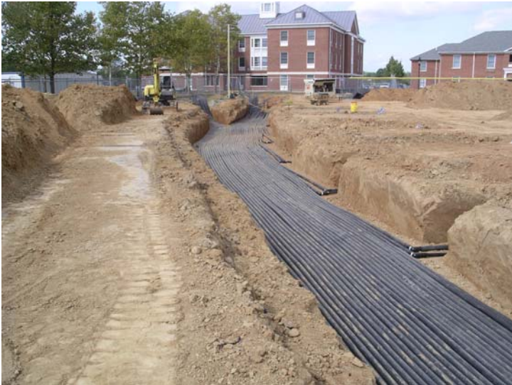
Photograph #2: Geothermal Trench Mains
