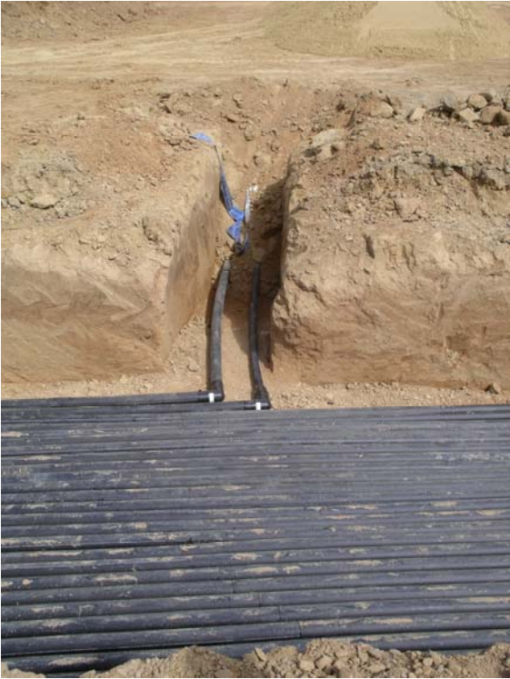
Photograph #5: Geothermal Circuit and Tracer Tape
