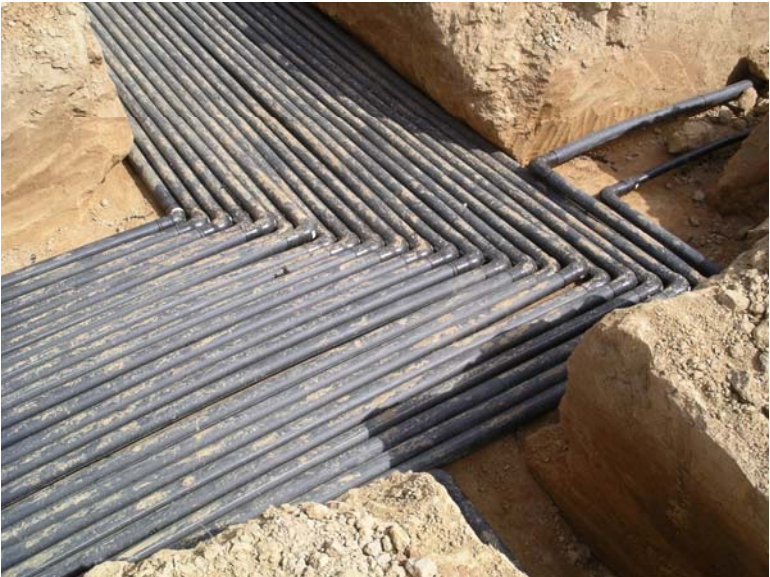
Photograph #4: Geothermal Fittings
