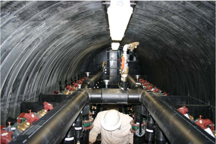
Photograph #6: Geothermal Vault Piping
